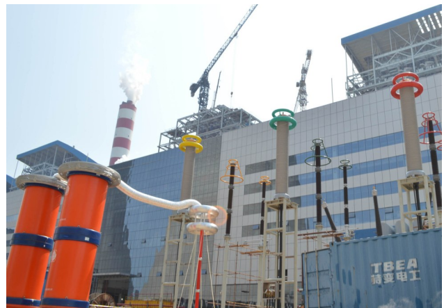
TBEA completes China's first domestically-made 500kV cables+accessories+construction integration project - 500kV XLPE insulated power cable project of the Shandong Chiping Xinfu 700MW generator set.
