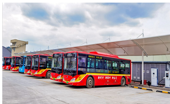
A TBEA charging station in Wuzhou
