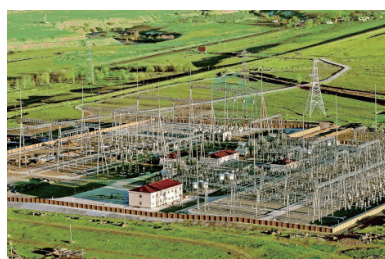
The 2x150MW Renovation and Expansion Project of the Bishkek Thermal Power Station in Kyrgyzstan won the 2019 China Power Quality Project Award.
