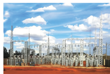
Phase I and II of the Nairobi 220kV and 66kV Power Grid Upgrading Project in Kenya
