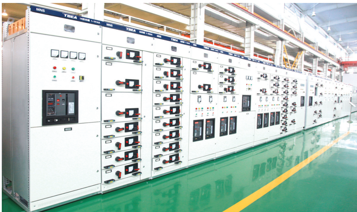
The MNS LV withdrawable switchgear cabinet used in the Changle Power Plant Project (First phase, 2×1000MW) constructed by Gansu Province Electric Power Investment Group Co., Ltd.
