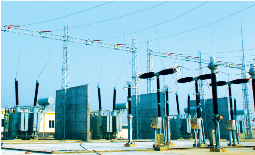
The world's first 330kV AT power supply traction transformer is used in the Zhengzhou-Xi'an Passenger Railway.
