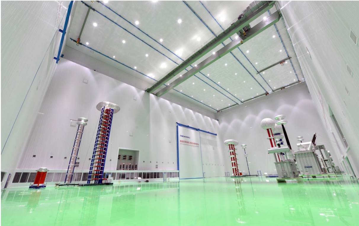
The world's first \pm 1100\text{kV} UHV transformer lab
