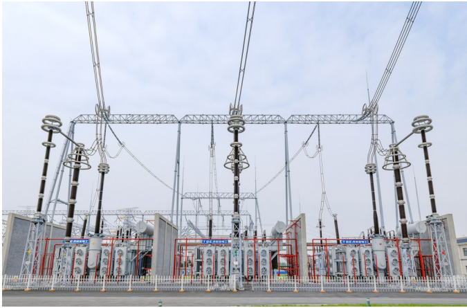
The world's first 1000kV power transformer and shunt reactor, independently developed by TBEA, is used in the world's first commercial 1000kV Southeast Shanxi-Nanyang-Jingmen UHV Alternative Current Test Demonstration Project. TBEA's UHV AC transmission critical technology, complete equipment and engineering application project won the National Science and Technology Progress Special Award.
