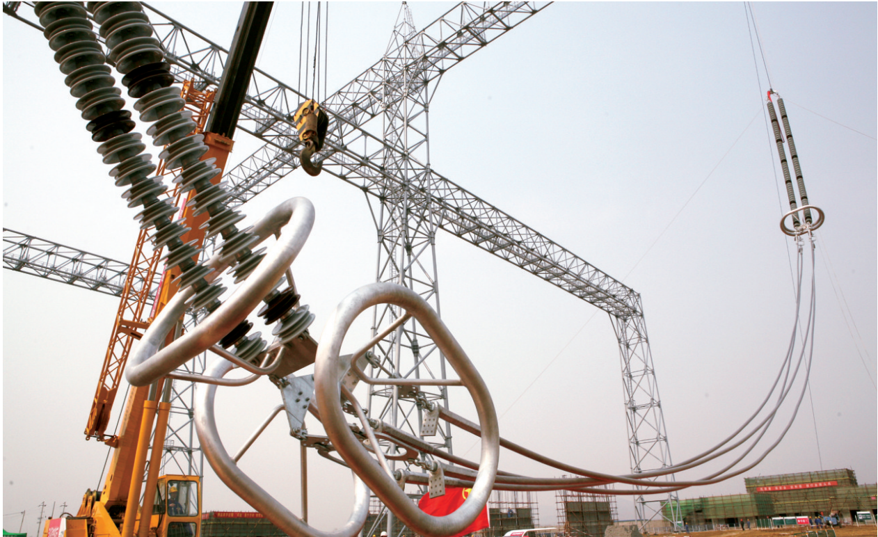
A large cross-section expanded diameter thermal-resistant aluminum alloy busbar is successfully operated in China's first UHV AC Project - 1000kV Southeast Shanxi-Nanyang-Jingmen UHV Alternative Current Test Demonstration Project.
