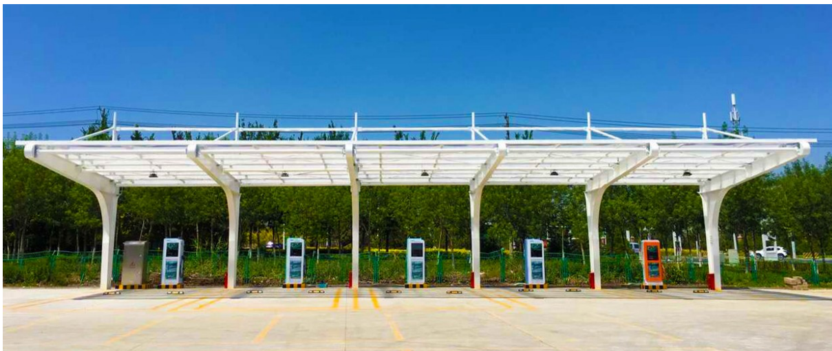
A TBEA charging station in Changji
