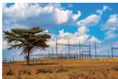
WOLAITA-AKAKI 400kV Transmission Project in Ethiopia.
