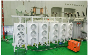
TBEA's DFP-700000/500 nuclear power transformer is used in the Taishan Nuclear Power Plant of CGN Power Co., Ltd., which boasts the world's largest unit capacity of its kind.
