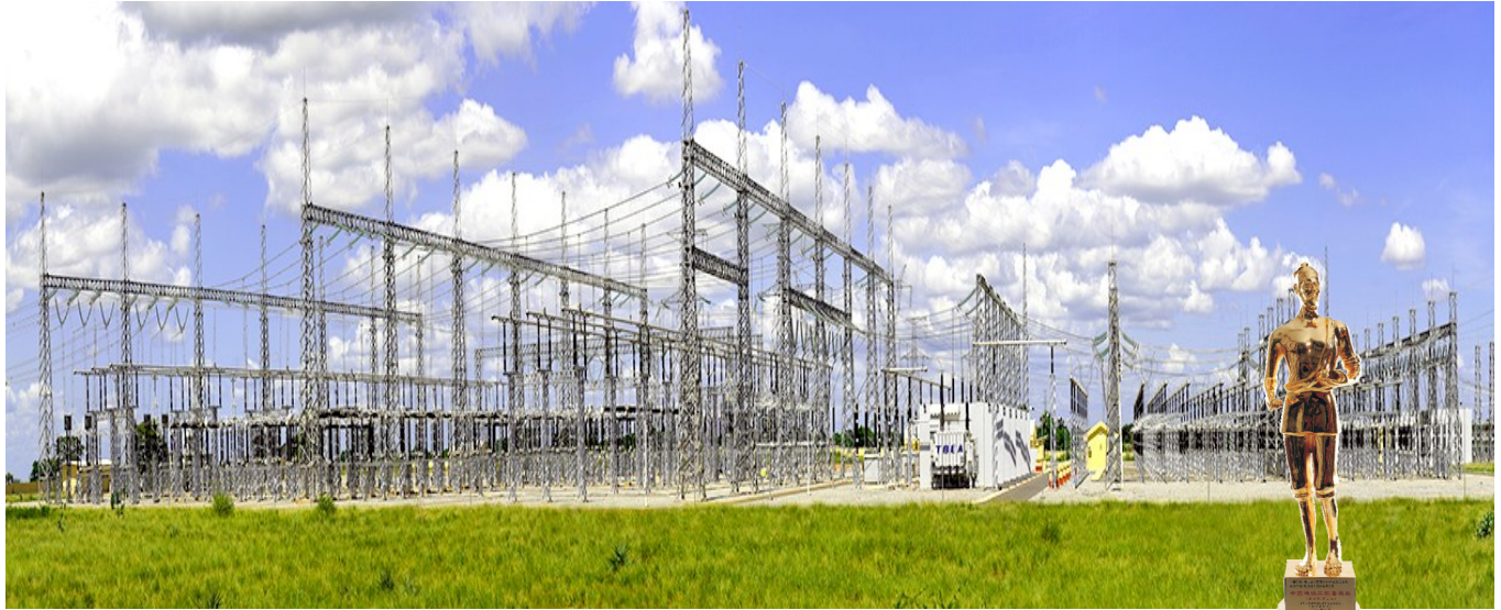
The Angola Soyo-Kapary Substation, one of TBEA's major overseas projects, was awarded the China Construction Engineering Luban Prize (Overseas Project), China's top construction award.
