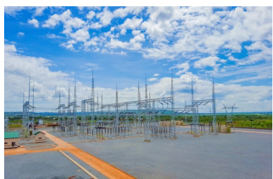
A photo of the Jatikalan Substation and the 765kV UHV Main Power Grid Transmission Project in India.
