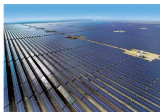
The 100MW PV Power Station in Punjab, Pakistan.
