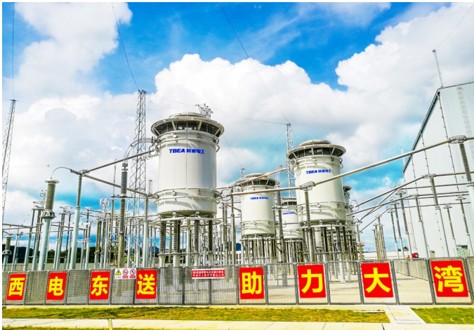
The world's first \pm 800\text{kV} dry hollow bridge arm reactor, independently developed by TBEA, is used at the receiving end of the Longmen Station of the Wudongde-Guangdong Guangxi UHV Multi Terminal Direct Current Demonstration Project. It boasts the world's highest voltage level and the largest AC/DC mixed current dry hollow bridge arm reactor.
