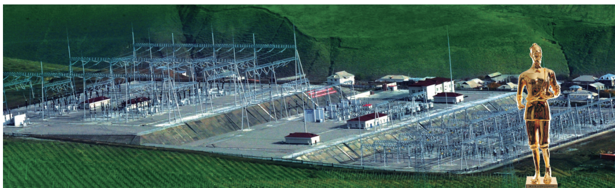
The Dushanbe 500kV Substation in Tajikistan won the China Construction Engineering Luban Prize (Overseas Project), China's top construction award.
